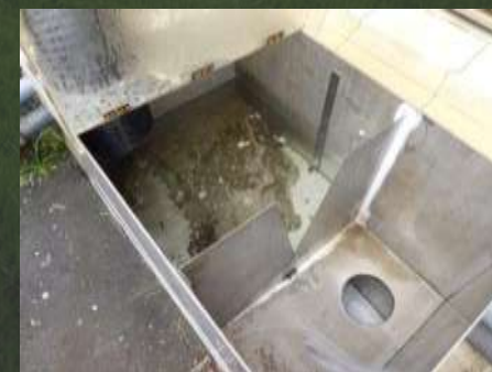
V-notch chamber receiving runoff from the control roof
