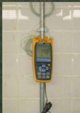
Thermocouple and data logger
