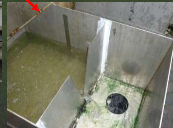
V-notch weir chamber
