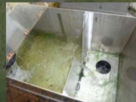
V-notch chamber receiving runoff from a green roof
